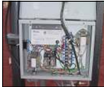
ELECTRONIC CONTROL IS USED TO KEEP THE TP CAN OIL/WATER AT BEST SEPARATION TEMPERATURE AND TO AUTO IGNITE THE PILOT ON THE INTEGRATED PROPANE BURNER
